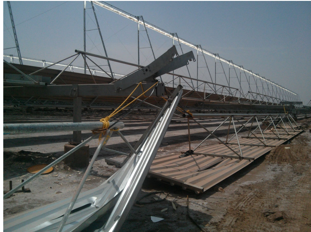
Solar Panels Destroyed by Wind
