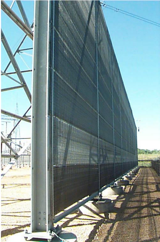
Transformer Station Wind Fence
